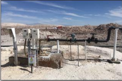
a) Brine production wells with surface equipment
