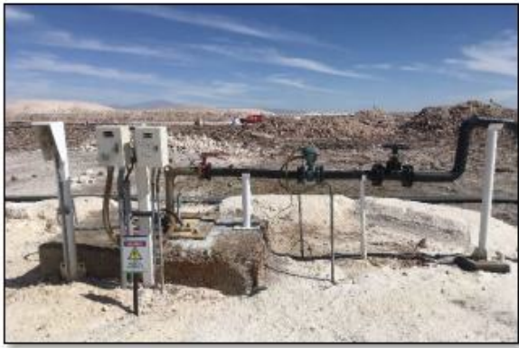
a) Brine production wells with surface equipment
