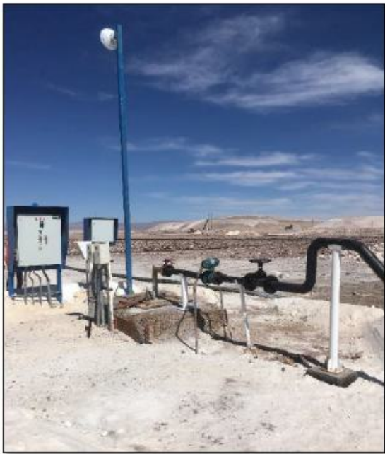
c) General view of a production brine well with an additional system for monitoring and control (telemetry)
