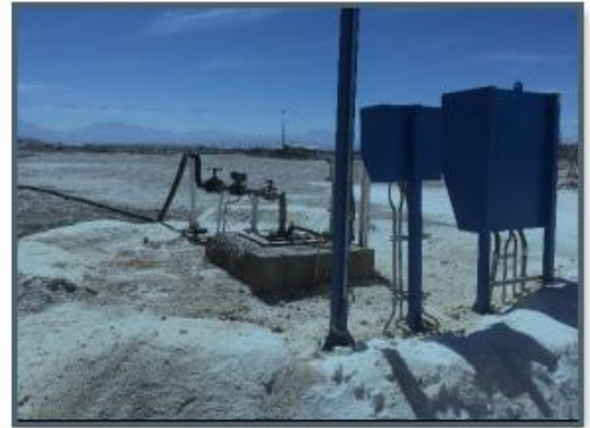
b) General view - production brine well and HDPE pipe for directing brine to the homogenization ponds
