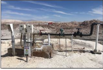
a) Brine production wells with surface equipment
